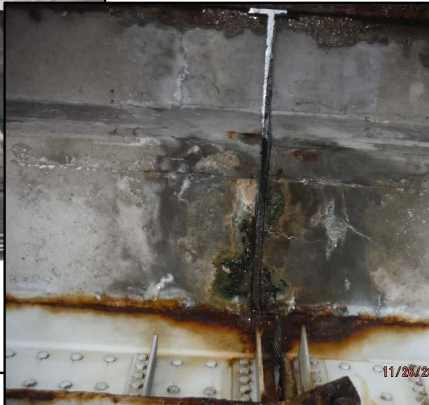
Looking up @ failed expansion Joint
